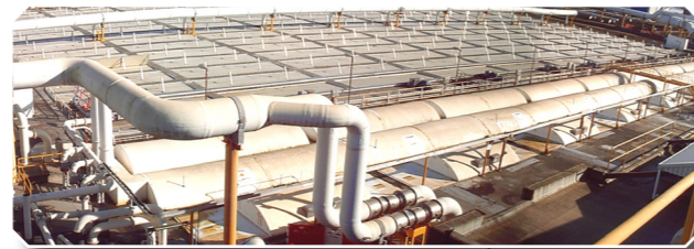
Primary sedimentation tanks
