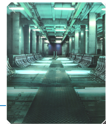
Inside the ultra violet (UV) treatment plant
