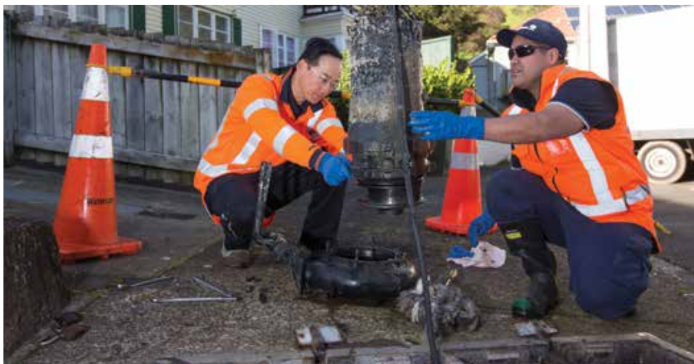
Maintenance servicemen Rick Yu (left) and Jim Burkhardt remove rags and wipes that were preventing a pump from pushing wastewater through the network.
