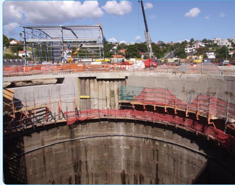
The permanent shaft, pictured in the forefront, will have a 1.4 metre deep base slab of concrete
