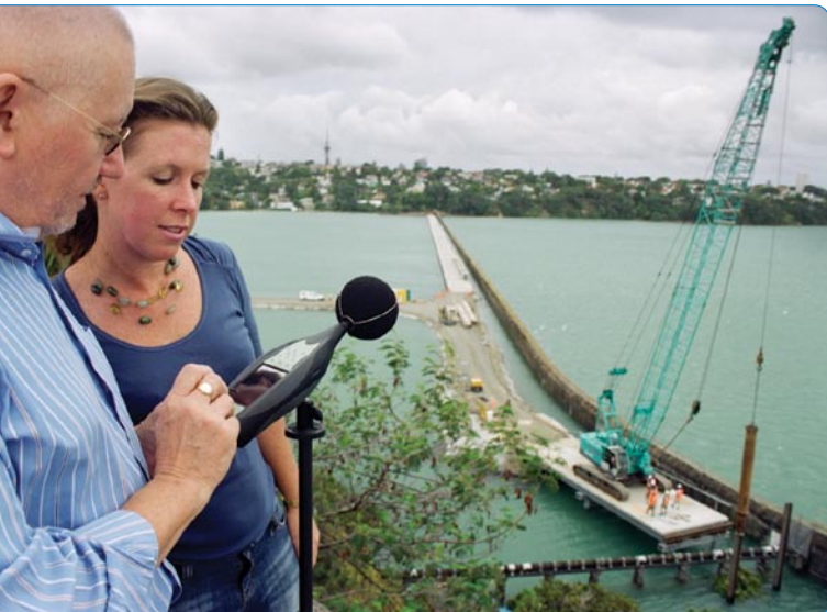
Environmental Planner Jenny Vince and Environmental Acoustic Consultant Michael Riley of J.P. Styles Ltd ensure the construction noise on the trestle way is within resource consent limits
