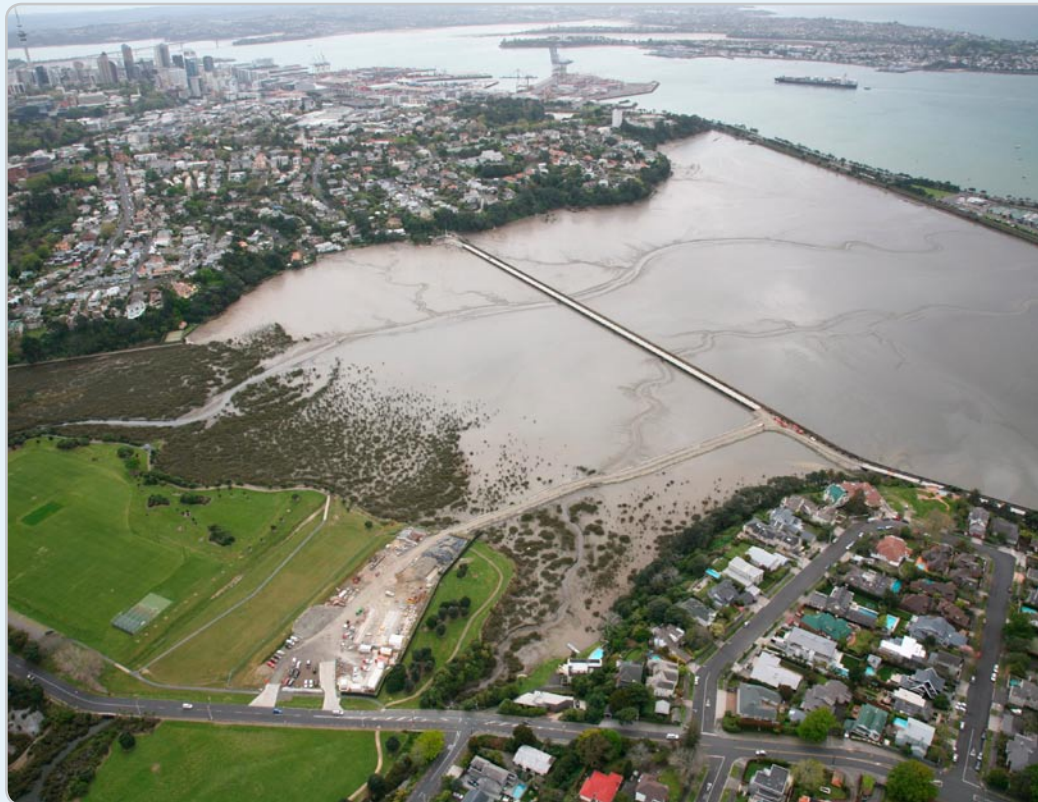
Aerial view showing the Shore Road construction site with the causeway and trestle way along the existing sewer to the bottom of Logan Terrace and Victoria Avenue.
