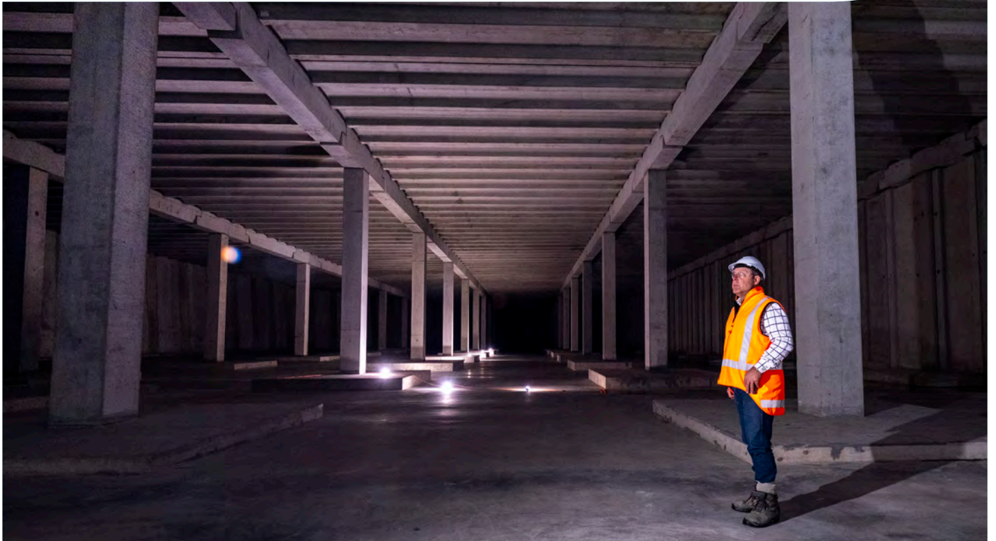
Watercare project manager Martin Hughes inside the newly constructed reservoir at our Redoubt Road complex.
